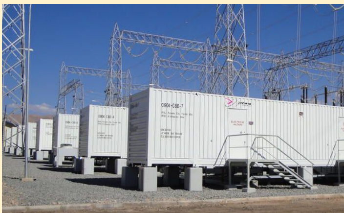
Future image of the ZPower Power Plant
